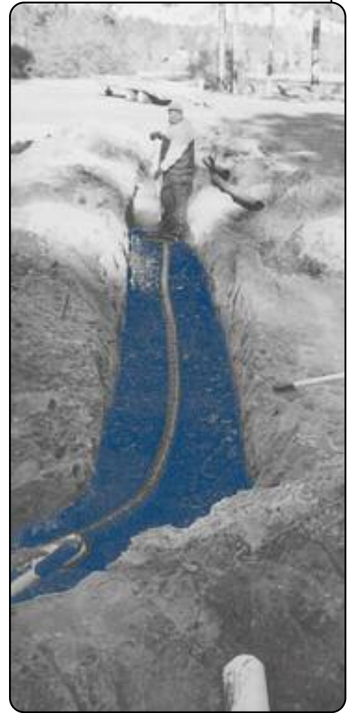
Bottom layer of trench with six inches of tire chips and four-inch pipe.
